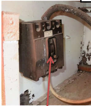
Battery Switch/Breaker On Left Side of Battery Compartment
